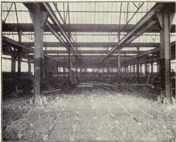
FIG. 36. INTERIOR OF MACHINE AND ERECTING DEPARTMENTS. CINCINNATI BICKFORD TOOL COMPANY.
